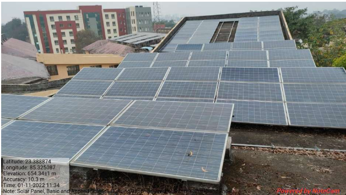
Fig. Solar Panel installed at Basic and Applied Science Building, Ranchi University, Ranchi
