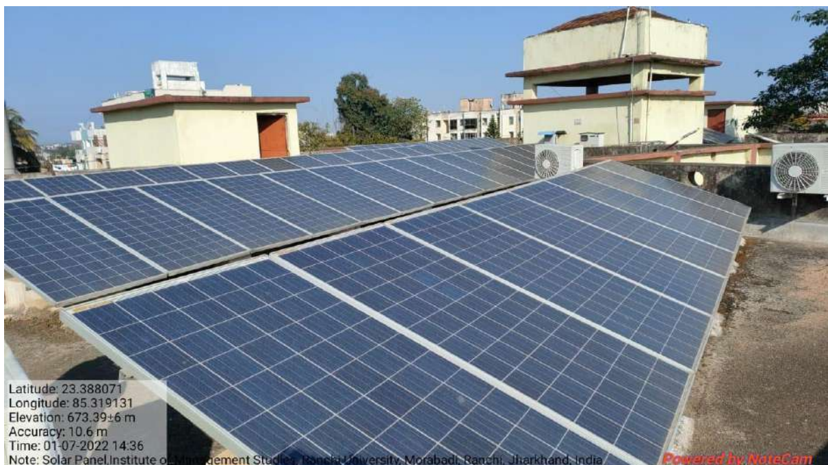
Fig. Solar Panel installed at IMS, Ranchi University, Ranchi
