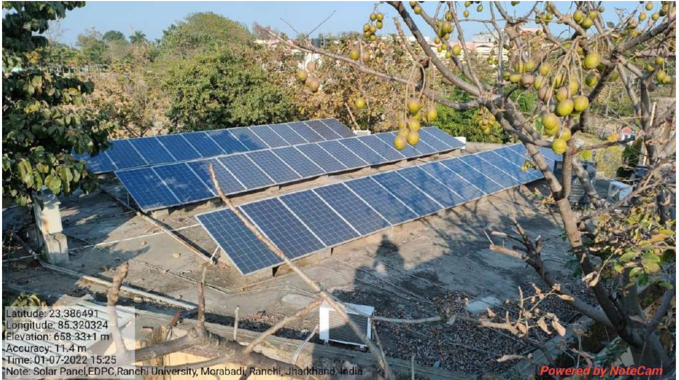
Fig. Solar Panel installed at EDPC, Examination Department, Ranchi University, Ranchi
