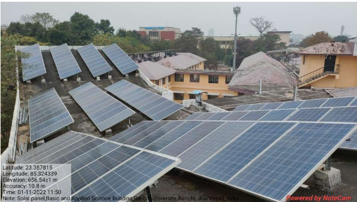
Fig. Solar Panel installed at Basic and Applied Science Building, Ranchi University, Ranchi
