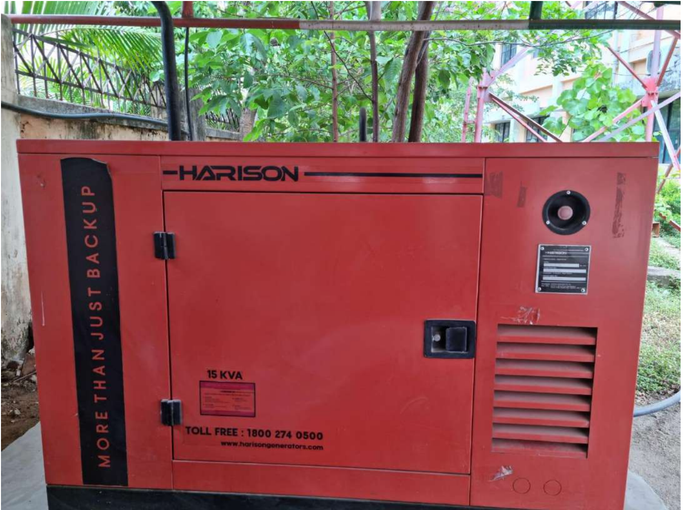
Fig. Silent Generator installed in the campus of Ranchi University, Ranchi.
