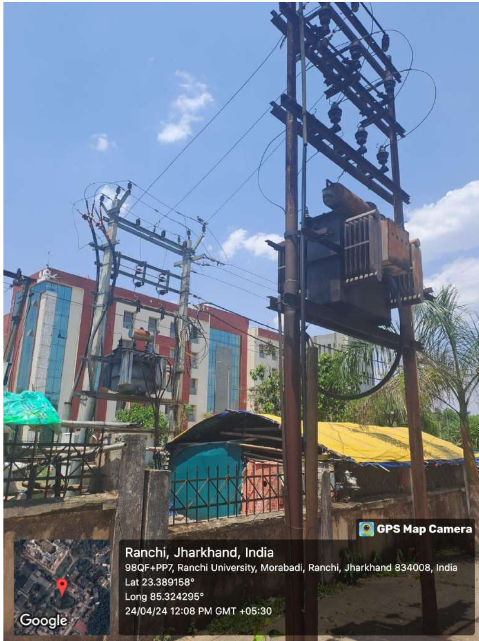
Fig. Electric Transformer installed at Basic and Applied Science Building, Ranchi University, Ranchi
