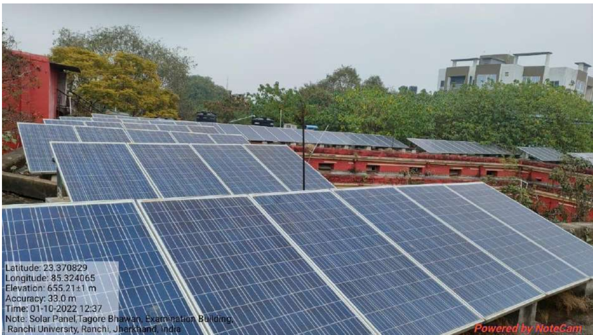
Fig. Solar Panel installed at Tagore Bhawan, Administrative Block, Sahedd Chowk, Ranchi University, Ranchi
